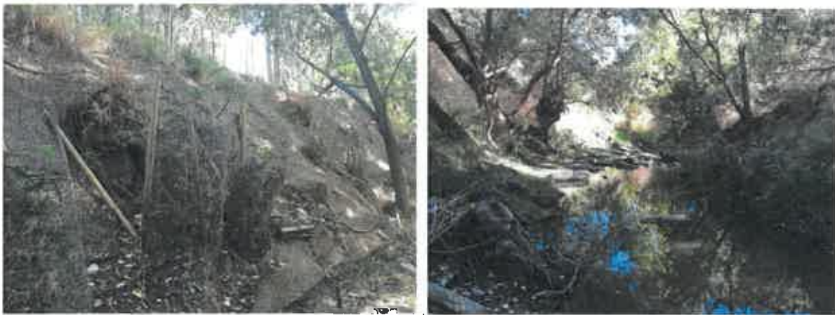
Some steep and unstable banks of San Lorenzo Creek
