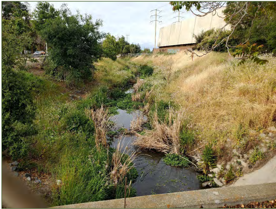
Photo 7. View of Mission Creek off site as it exits box culvert under Paseo Padre Parkway in a box heading southwest. Facing southwest. April 25, 2022.
