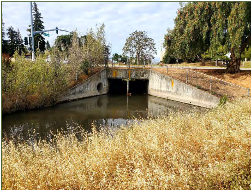
Photo 6. View of Mission Creek as it flows south off the site under Paseo Padre Parkway in a box culvert. Facing southwest. April 25, 2022.
