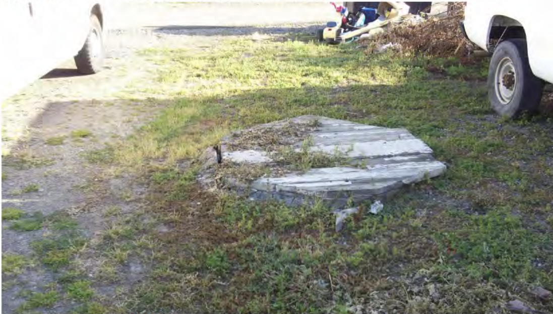
PHOTO 34. 16309 Kent Avenue – Damaged Wooden Cover of Water Cistern (sand filled) Located in Parking Area West of Unit 17
