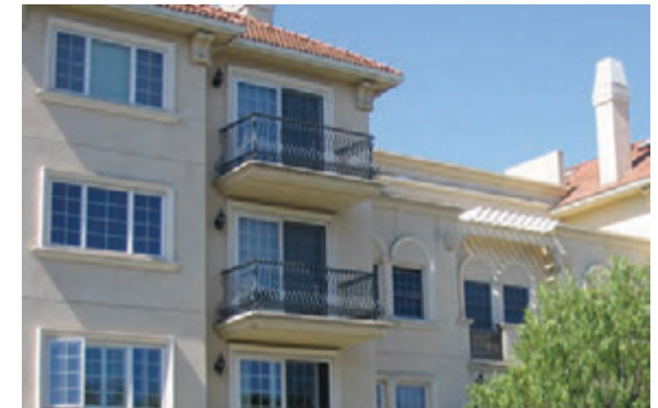
Although the windows on this facade differ in shape and size, the consistent use of trim style and windows with similarly space mullions help create a consistent look. (Guideline E-34)
