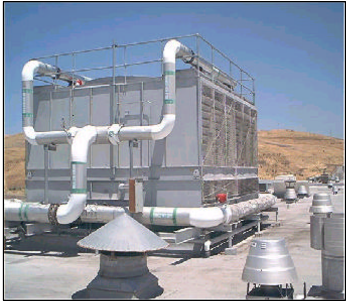
Modified central plant cooling tower installation features an 850-ton high efficiency chiller
