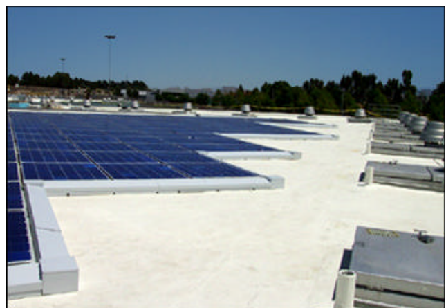
PowerGuard® Solar Electric System on the roof of the Santa Rita Jail with cool roof reflective coating.
