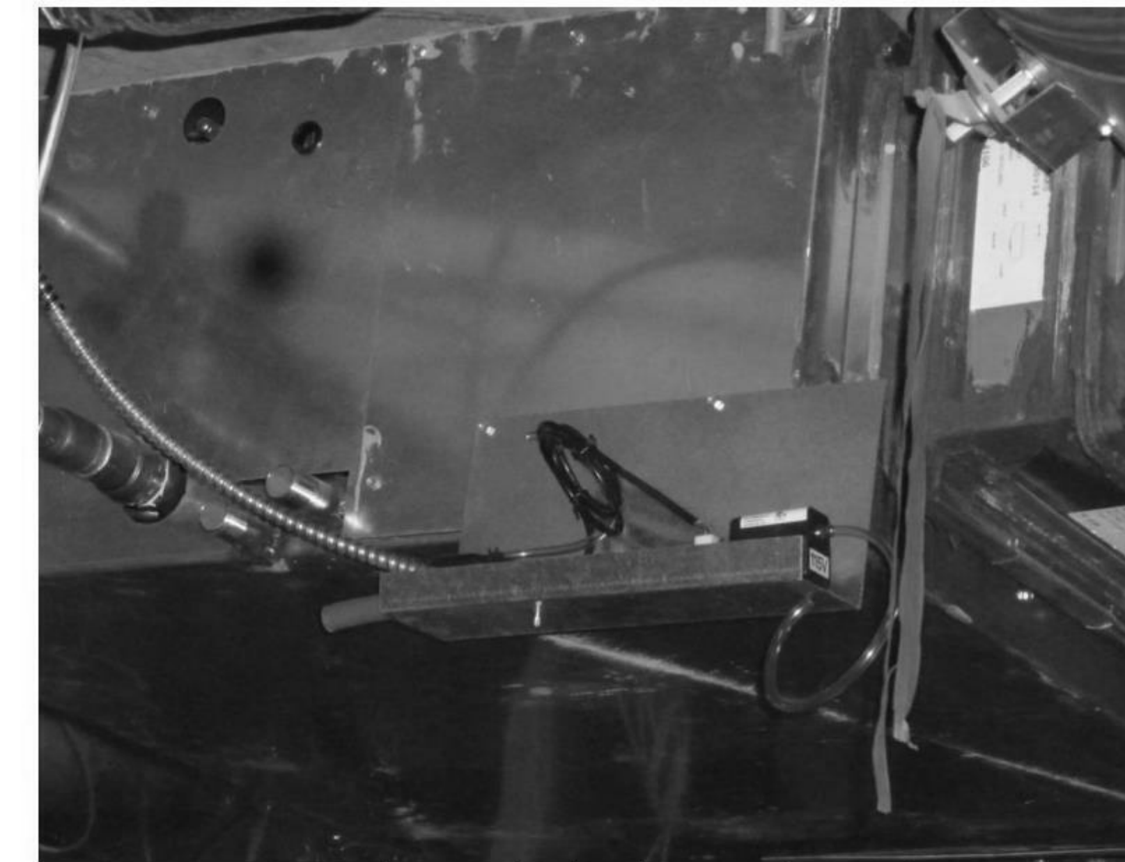
Figure 4: Condensate Pump for cooling coil downstream of VAV terminal
