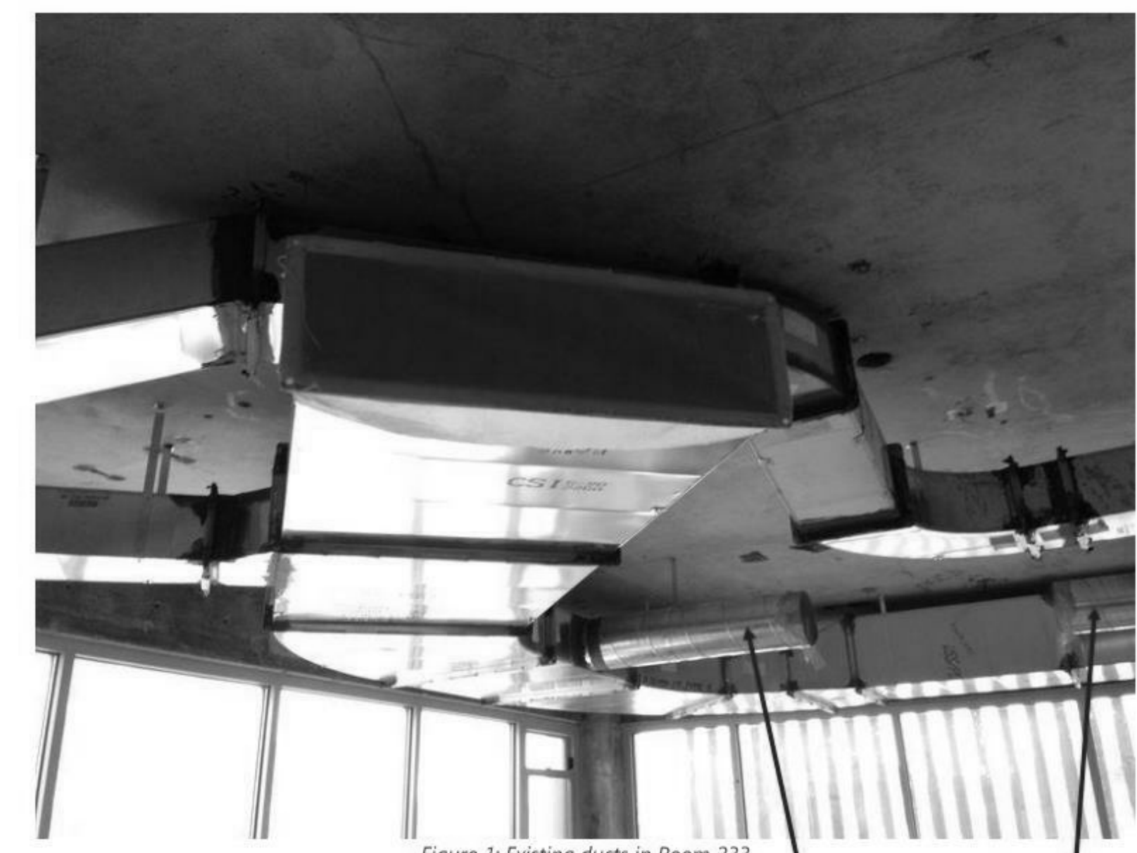
Figure 1: Existing ducts in Room 233
