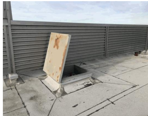
Item #: 525491 Uniformat Number: B3060 Item Title: Roof Hatches Caption: Roof hatch finish is deteriorating. Surface rust was observed. Roof hatch is missing railing Priority: 3 - Necessary - Not Yet Critical
