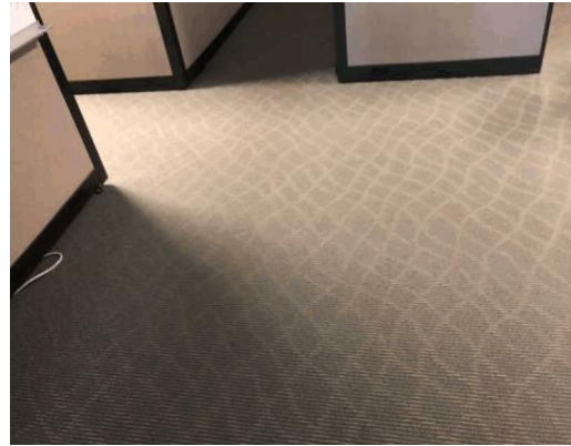
Item #: 525367 Uniformat Number: C2030 Item Title: Sheet Carpeting Caption: Flooring is stained and showing signs of wear. Priority: 4 - Recommended
