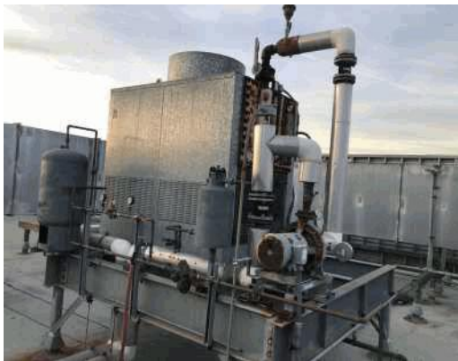
Item #: 493863 Uniformat Number: D3020 Item Title: Fuel-Fired Heating Boilers - 501 to 1750 MBH Caption: Hot water boiler Priority: 1 - Currently Critical
