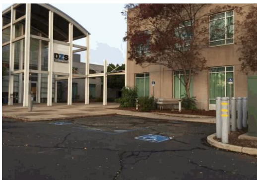
Item #: 489144 Uniformat Number: H2010 Item Title: ADA Assessments Caption: ADA-designated parking is non-compliant. The path of travel to the building entrance is not clearly marked and there is no loading zone at the parking space. Priority: 2 - Potentially Critical
