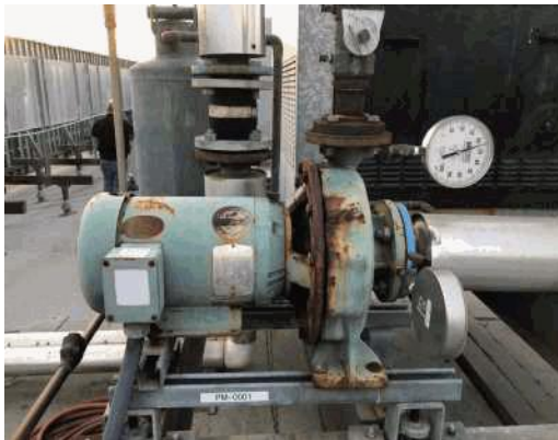
Item #: 493861 Uniformat Number: D3050 Item Title: Hot Water Pumps- 0 to 10 HP Caption: Hot water pump Priority: 2 - Potentially Critical
