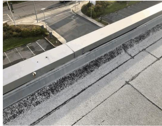
Item #: 525488 Uniformat Number: B3010 Item Title: Roofing - Unprotected Membrane Caption: Roof is approaching the the end of the expected life cycle Priority: 4 - Recommended
