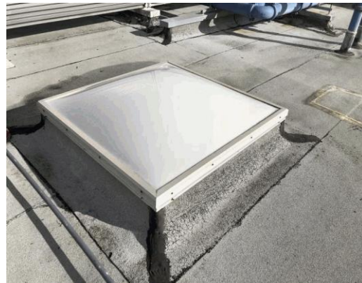
Item #: 525400 Uniformat Number: B3060 Item Title: Skylights Caption: Skylights do not have fall protection Priority: 2 - Potentially Critical
