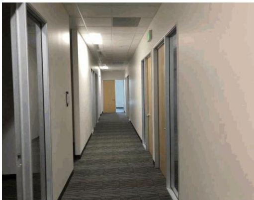
Item #: 525379 Uniformat Number: C2030 Item Title: Sheet Carpeting Caption: In other areas, the flooring is functional, but has exceeded the expected lifecycle. Priority: 3 - Necessary - Not Yet Critical
