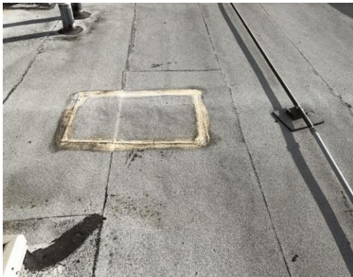
Item #: 525287 Uniformat Number: B3010 Item Title: Roofing - Unprotected Membrane Caption: Numerous roof patches were observed Priority: 4 - Recommended
