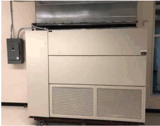
Item #: 493865 Uniformat Number: D3040 Item Title: Computer-Room Air-Conditioners Caption: Typical Computer room A/C unit Priority: 1 - Currently Critical
