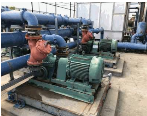
Item #: 493851 Uniformat Number: D3050 Item Title: Condenser Water Pumps- 11 TO 50 HP Caption: Condenser water pumps Priority: 3 - Necessary - Not Yet Critical
