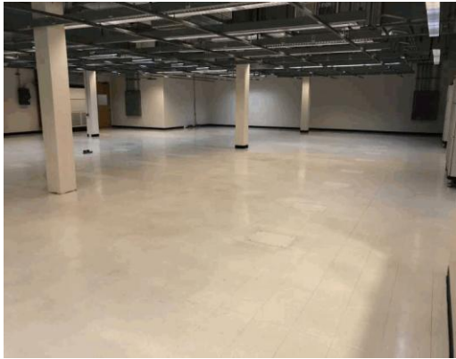
Item #: 525383 Uniformat Number: C2030 Item Title: Vinyl Composite Tile Flooring Caption: Flooring is damaged in some areas. Flooring has exceeded the lifecycle expectancy. Priority: 4 - Recommended
