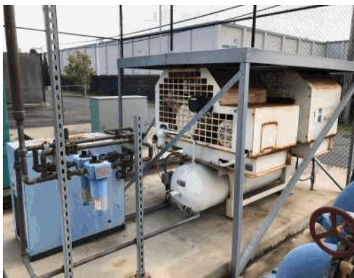
Item #: 493853 Uniformat Number: D2060 Item Title: Air Compressors - Duplex Caption: Air compressor & air dryer Priority: 3 - Necessary - Not Yet Critical
