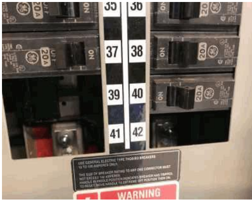
Item #: 493625 Uniformat Number: D5020 Item Title: Panelboard Deficiencies Caption: ZX5 Priority: 1 - Currently Critical
