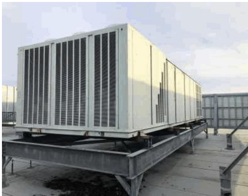
Item #: 493875 Uniformat Number: D3060 Item Title: Packaged DX Air-Conditioning Units- 6 to 50 TON Caption: Packaged DX Rooftop unit Priority: 1 - Currently Critical
