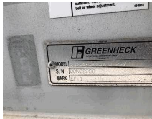
Item #: 493890 Uniformat Number: D3060 Item Title: Exhaust Air HVAC Fans- General Caption: EF-1 nameplate Priority: 1 - Currently Critical
