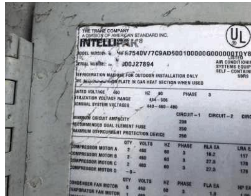
Item #: 493875 Uniformat Number: D3060 Item Title: Packaged DX Air-Conditioning Units- 6 to 50 TON Caption: Packaged DX Rooftop unit nameplate Priority: 1 - Currently Critical
