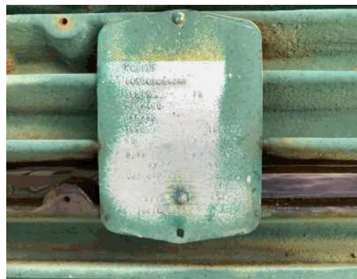
Item #: 493851 Uniformat Number: D3050 Item Title: Condenser Water Pumps- 11 TO 50 HP Caption: Condenser water pump Motor nameplate Priority: 3 - Necessary - Not Yet Critical
