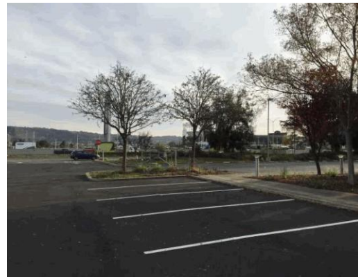
Item #: 489338 Uniformat Number: H2010 Item Title: ADA Assessments Caption: Parking spaces Priority: 1 - Currently Critical
