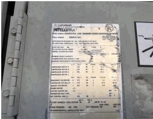
Item #: 493862 Uniformat Number: D3060 Item Title: Packaged DX Air-Conditioning Units- 6 to 50 TON Caption: RTU Nameplate Priority: 1 - Currently Critical
