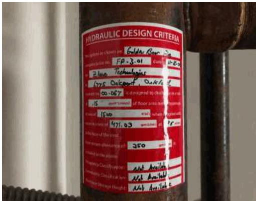
Item #: 493872 Uniformat Number: D4010 Item Title: Fire Suppression - Wet System Caption: Design placard Priority: 1 - Currently Critical
