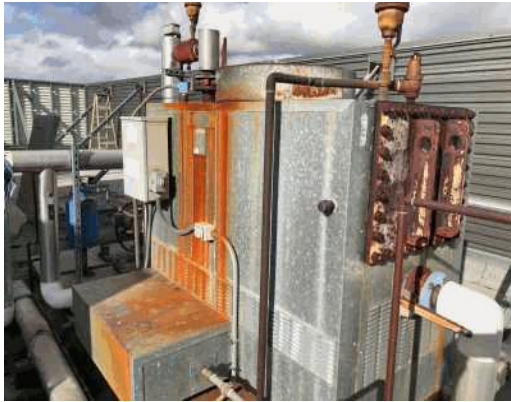
Item #: 493846 Uniformat Number: D3020 Item Title: Fuel-Fired Heating Boilers - 501 to 1750 MBH Caption: Hot water boiler Priority: 4 - Recommended
