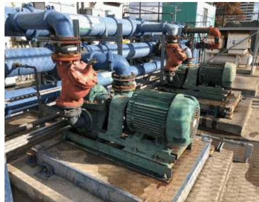
Item #: 493849 Uniformat Number: D3050 Item Title: Chilled Water Pumps- 11 TO 50 HP Caption: Chilled water pumps Priority: 3 - Necessary - Not Yet Critical
