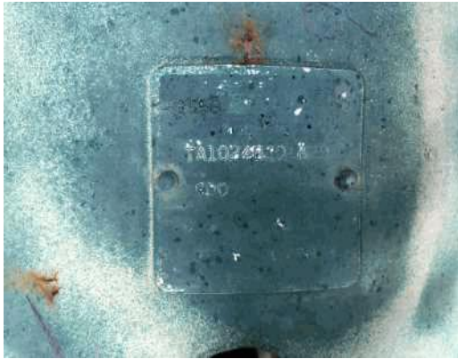
Item #: 493851 Uniformat Number: D3050 Item Title: Condenser Water Pumps- 11 TO 50 HP Caption: Condenser water pump nameplate Priority: 3 - Necessary - Not Yet Critical
