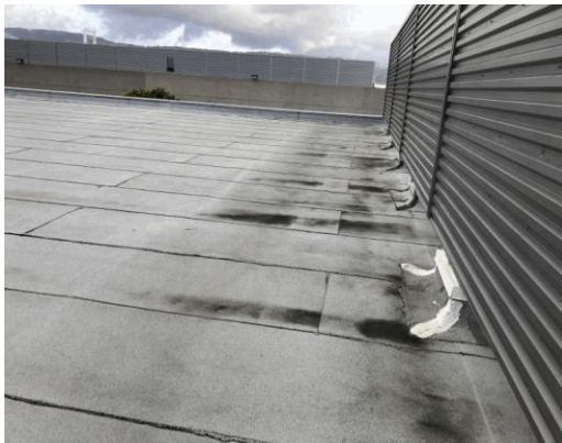
Item #: 525287 Uniformat Number: B3010 Item Title: Roofing - Unprotected Membrane Caption: View of aging roof system Priority: 4 - Recommended
