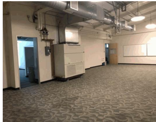
Item #: 525379 Uniformat Number: C2030 Item Title: Sheet Carpeting Caption: Flooring is stained and showing signs of wear in some areas Priority: 3 - Necessary - Not Yet Critical
