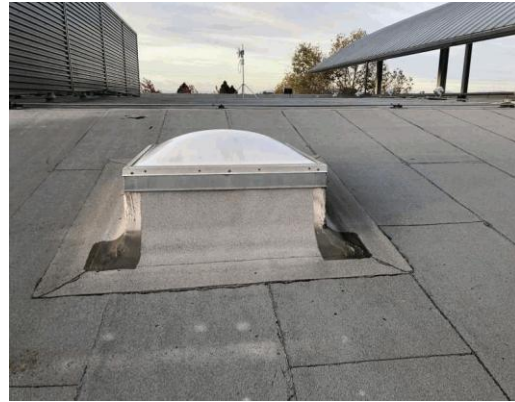
Item #: 525387 Uniformat Number: B3060 Item Title: Skylights Caption: Skylights do not have fall protection Priority: 3 - Necessary - Not Yet Critical
