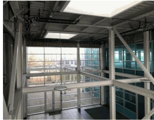
Item #: 525530 Uniformat Number: B2010 Item Title: Exterior Curtain Wall Assemblies Caption: Energy inefficient single-pane glazed curtain wall assemblies Priority: 3 - Necessary - Not Yet Critical
