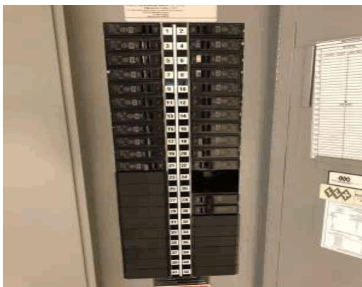
Item #: 493625 Uniformat Number: D5020 Item Title: Panelboard Deficiencies Caption: ZX3A Priority: 1 - Currently Critical
