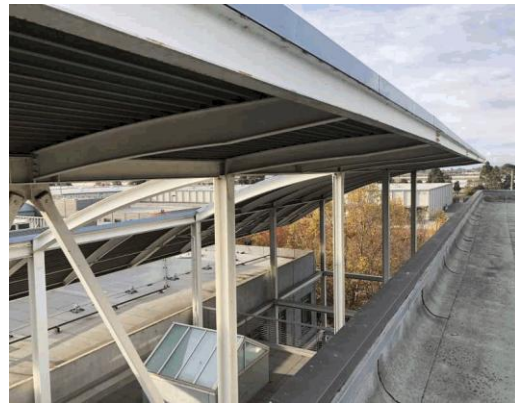
Item #: 525529 Uniformat Number: B1030 Item Title: Steel Building Structure Caption: Areas of the steel canopy frame is beginning to rust Priority: 3 - Necessary - Not Yet Critical
