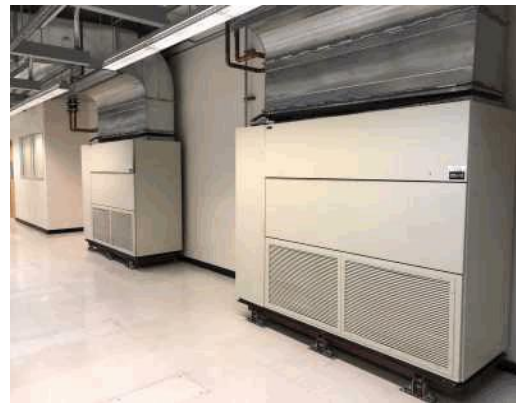
Item #: 493865 Uniformat Number: D3040 Item Title: Computer-Room Air-Conditioners Caption: Water cooled Computer room A/C units Priority: 1 - Currently Critical
