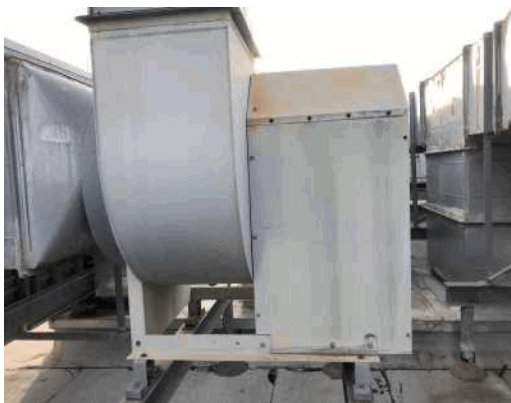
Item #: 493890 Uniformat Number: D3060 Item Title: Exhaust Air HVAC Fans- General Caption: EF-1 Priority: 1 - Currently Critical
