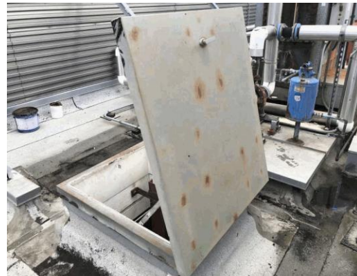
Item #: 525345 Uniformat Number: B3060 Item Title: Roof Hatches Caption: Roof hatch finish is deteriorating. Surface rust was observed. Roof hatch is missing railing Priority: 3 - Necessary - Not Yet Critical
