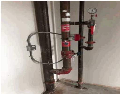
Item #: 493872 Uniformat Number: D4010 Item Title: Fire Suppression - Wet System Caption: Interior standpipe riser Priority: 1 - Currently Critical
