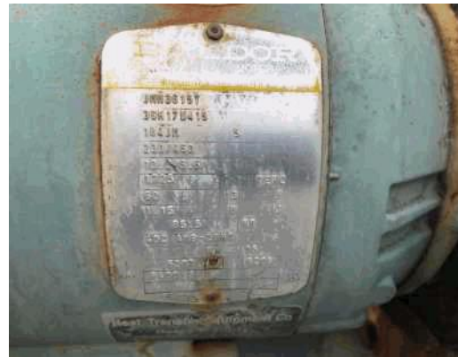
Item #: 493861 Uniformat Number: D3050 Item Title: Hot Water Pumps- 0 to 10 HP Caption: Hot water pump motor nameplate Priority: 2 - Potentially Critical
