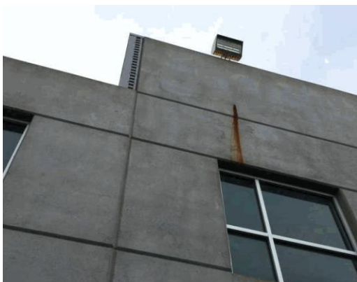
Item #: 489155 Uniformat Number: B2010 Item Title: Exterior Walls Caption: Corrosion at exterior wall Priority: 2 - Potentially Critical
