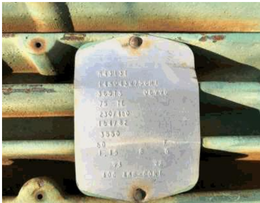
Item #: 493849 Uniformat Number: D3050 Item Title: Chilled Water Pumps- 11 TO 50 HP Caption: Pump motor nameplate Priority: 3 - Necessary - Not Yet Critical
