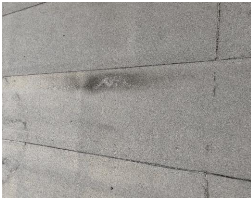
Item #: 525384 Uniformat Number: B3010 Item Title: Roofing - Unprotected Membrane Caption: Roof is approaching the the end of the expected life cycle Priority: 4 - Recommended
