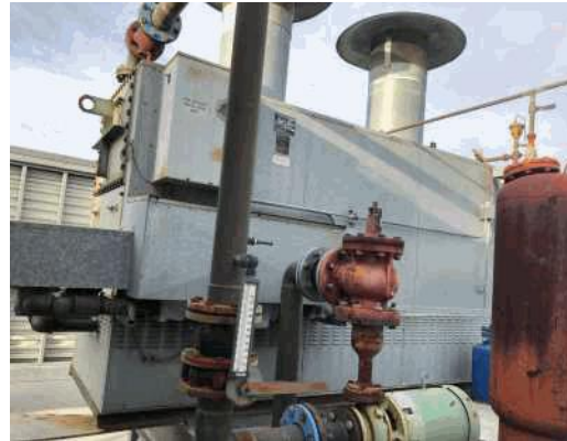
Item #: 493889 Uniformat Number: D3020 Item Title: Fuel-Fired Heating Boilers - 3751 to 7500 MBH Caption: Hot water boiler Priority: 1 - Currently Critical
