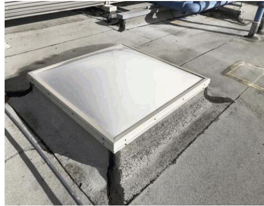
Item #: 525287 Uniformat Number: B3010 Item Title: Roofing - Unprotected Membrane Caption: Roof membrane at roof curbs and parapets are beginning to crack & deteriorate. Priority: 4 - Recommended
