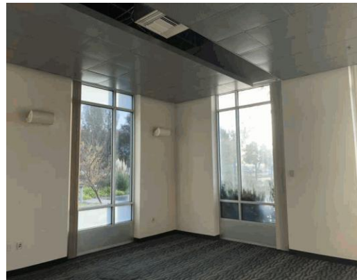
Item #: 525410 Uniformat Number: B2020 Item Title: Aluminum Windows (fixed) Caption: Energy inefficient single pane glazing assemblies observed Priority: 3 - Necessary - Not Yet Critical
