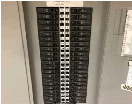
Item #: 493474 Uniformat Number: D5020 Item Title: Electrical Arc Flash Hazard Analysis and Short Circuit Coordination Caption: Equipment not labeled with hazards Priority: 1 - Currently Critical
