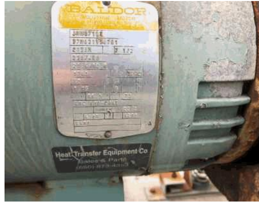
Item #: 493845 Uniformat Number: D3050 Item Title: Hot Water Pumps- 0 to 10 HP Caption: Hot water pump motor nameplate Priority: 2 - Potentially Critical
