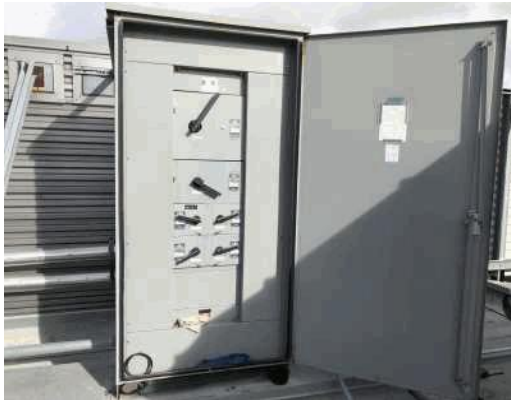
Item #: 493479 Uniformat Number: D5020 Item Title: Electrical Arc Flash Hazard Analysis and Short Circuit Coordination Caption: Equipment not labeled with required safety information Priority: 1 - Currently Critical
