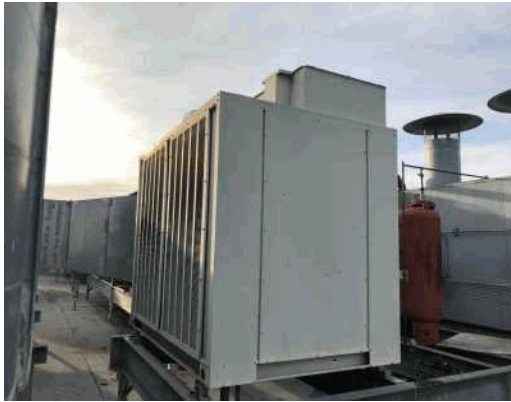
Item #: 493888 Uniformat Number: D3040 Item Title: Split-System Air-Conditioners Caption: Air cooled condenser section Priority: 1 - Currently Critical
