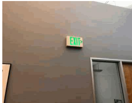
Item #: 493495 Uniformat Number: D5040 Item Title: Exit Signs Caption: Exit sign Priority: 1 - Currently Critical
