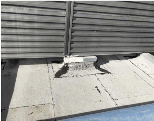
Item #: 525287 Uniformat Number: B3010 Item Title: Roofing - Unprotected Membrane Caption: Roof membrane at roof curbs and parapets are beginning to crack & deteriorat Priority: 4 - Recommended
