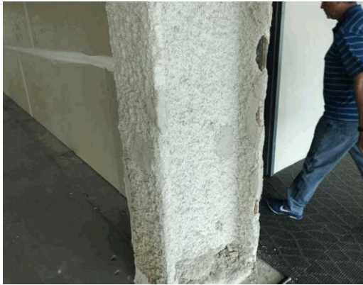
Item #: 525465 Uniformat Number: B1030 Item Title: Steel Building Structure Caption: Some fireproofing on steel columns is missing Priority: 3 - Necessary - Not Yet Critical
