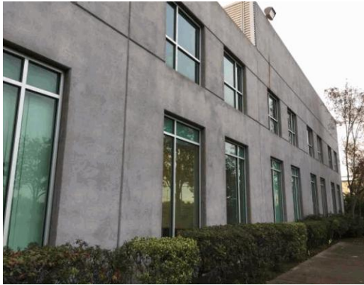
Item #: 489210 Uniformat Number: B2020 Item Title: Exterior Windows Caption: Energy inefficient single pane glazing assemblies observed Priority: 2 - Potentially Critical
