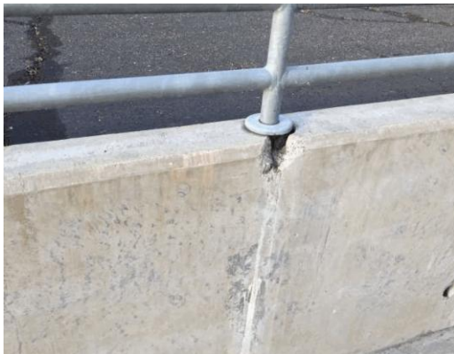
Item #: 489215 Uniformat Number: G2030 Item Title: Exterior Concrete Ramps Caption: Concrete wall at loading dock ramp 1 Priority: 2 - Potentially Critical
