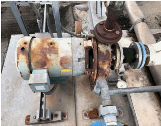
Item #: 493845 Uniformat Number: D3050 Item Title: Hot Water Pumps- 0 to 10 HP Caption: Hot water pump Priority: 2 - Potentially Critical
