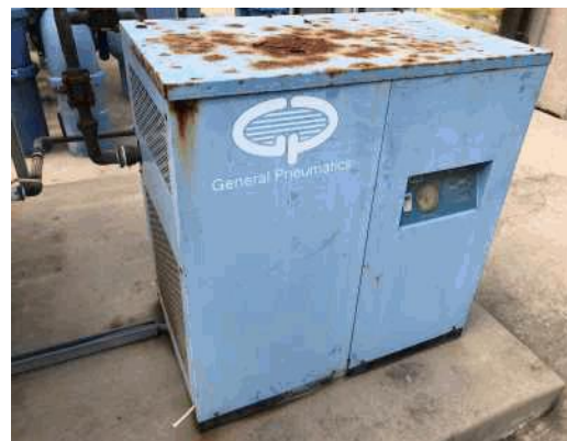
Item #: 493853 Uniformat Number: D2060 Item Title: Air Compressors - Duplex Caption: Air dryer Priority: 3 - Necessary - Not Yet Critical
