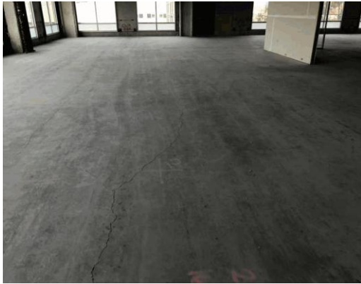
Item #: 525456 Uniformat Number: B1010 Item Title: Composite Floor Decking Caption: Surface cracking in concrete topping was observed. Priority: 4 - Recommended
