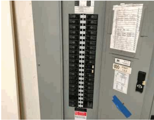
Item #: 493498 Uniformat Number: D5020 Item Title: Electrical Service And Distribution Caption: Panel L1B Priority: 1 - Currently Critical
