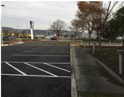
Item #: 489217 Uniformat Number: H2010 Item Title: ADA Assessments Caption: Non compliant parking space Priority: 2 - Potentially Critical
