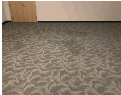
Item #: 525382 Uniformat Number: C2030 Item Title: Sheet Carpeting Caption: Flooring is stained and showing signs of wear Priority: 3 - Necessary - Not Yet Critical
