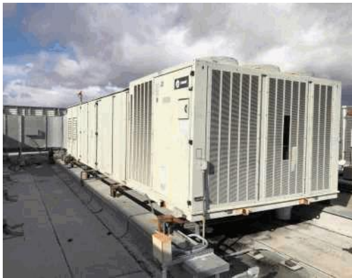
Item #: 493838 Uniformat Number: D3060 Item Title: Packaged DX Air-Conditioning Units- 6 to 50 TON Caption: 60 Ton A/C unit Priority: 4 - Recommended
