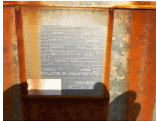
Item #: 493846 Uniformat Number: D3020 Item Title: Fuel-Fired Heating Boilers - 501 to 1750 MBH Caption: Hot water boiler nameplate Priority: 4 - Recommended
