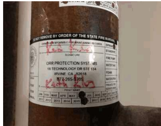
Item #: 493872 Uniformat Number: D4010 Item Title: Fire Suppression - Wet System Caption: Out of date inspection sticker Priority: 1 - Currently Critical
