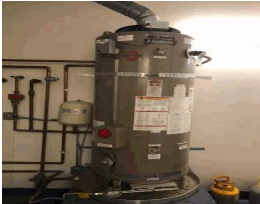
Item #: 493864 Uniformat Number: D2010 Item Title: Domestic Water Heaters Caption: Gas hot water heater Priority: 1 - Currently Critical
