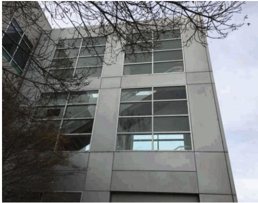
Item #: 490815 Uniformat Number: B2010 Item Title: Exterior Walls Caption: Staining observed on exterior walls Priority: 3 - Necessary - Not Yet Critical
