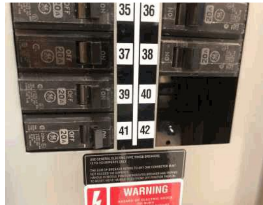
Item #: 493498 Uniformat Number: D5020 Item Title: Electrical Service And Distribution Caption: Empty circuit breakers location Priority: 1 - Currently Critical
