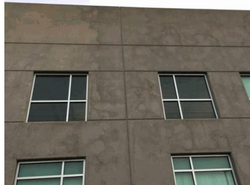
Item #: 489155 Uniformat Number: B2010 Item Title: Exterior Walls Caption: Cracking in concrete walls Priority: 2 - Potentially Critical
