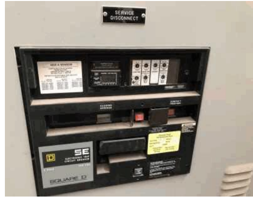
Item #: 493498 Uniformat Number: D5020 Item Title: Electrical Service And Distribution Caption: Switchboard MSB Priority: 1 - Currently Critical
