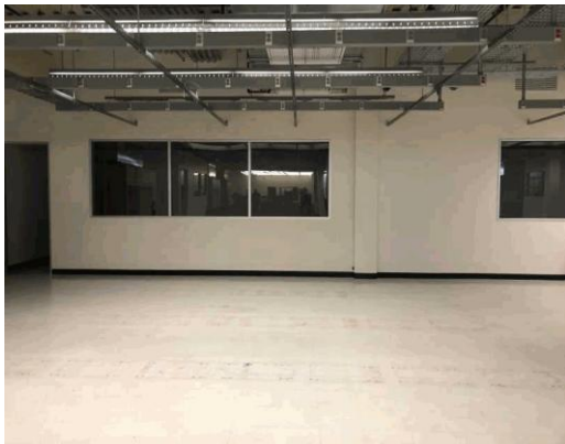
Item #: 525381 Uniformat Number: C2030 Item Title: Vinyl Composite Tile Flooring Caption: Flooring is damaged in some areas. Flooring has exceeded the lifecycle expectancy. Priority: 4 - Recommended
