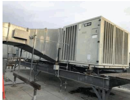
Item #: 493862 Uniformat Number: D3060 Item Title: Packaged DX Air-Conditioning Units- 6 to 50 TON Caption: Packaged DX Rooftop unit Priority: 1 - Currently Critical
