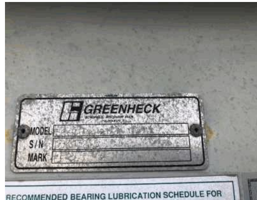
Item #: 493890 Uniformat Number: D3060 Item Title: Exhaust Air HVAC Fans- General Caption: E-2 nameplate Priority: 1 - Currently Critical
