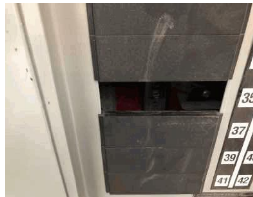
Item #: 493498 Uniformat Number: D5020 Item Title: Electrical Service And Distribution Caption: Empty circuit breaker location Priority: 1 - Currently Critical
