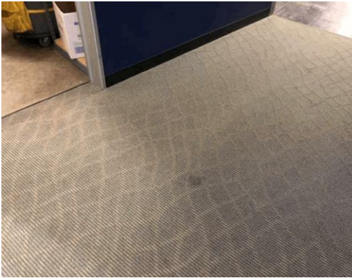
Item #: 525211 Uniformat Number: C2030 Item Title: Sheet Carpeting Caption: Flooring is stained and showing signs of wear Priority: 4 - Recommended
