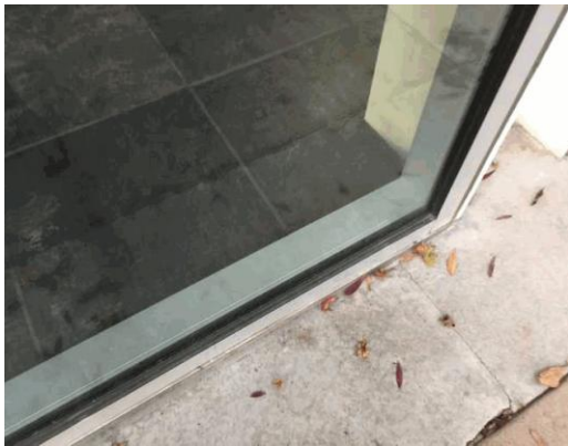
Item #: 489208 Uniformat Number: B2020 Item Title: Storefronts Caption: Energy inefficient single pane glazing assemblies observed Priority: 2 - Potentially Critical
