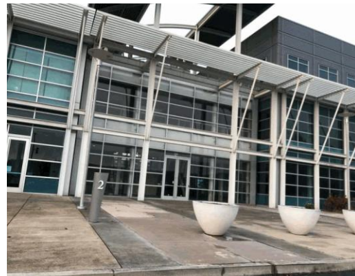
Item #: 525408 Uniformat Number: B2010 Item Title: Exterior Curtain Wall Assemblies Caption: Energy inefficient single pane glazing Priority: 3 - Necessary - Not Yet Critical
