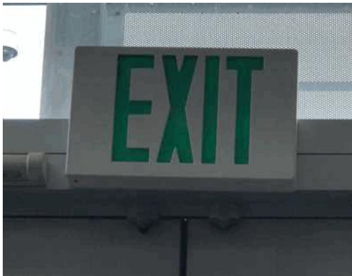
Item #: 493495 Uniformat Number: D5040 Item Title: Exit Signs Caption: Inoperable exit sign Priority: 1 - Currently Critical
