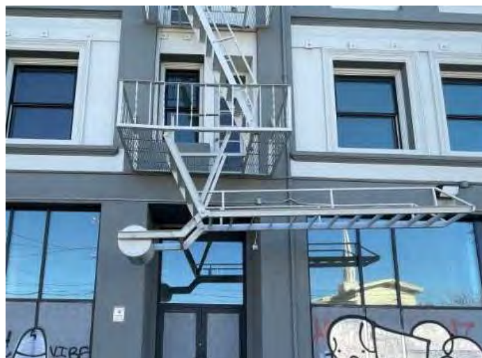
96. Certification and making the fire escape safe is required
