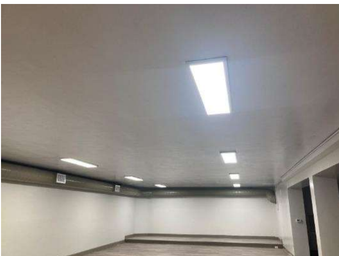
59. LED lighting in the basement
