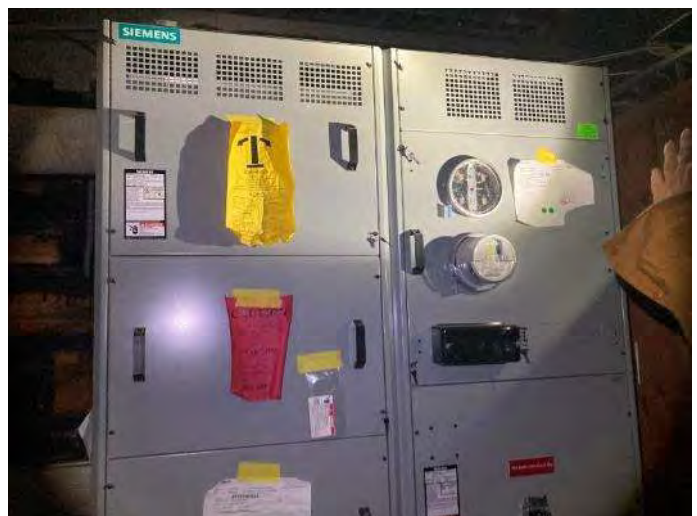
48. Electrical switchboard in the basement
