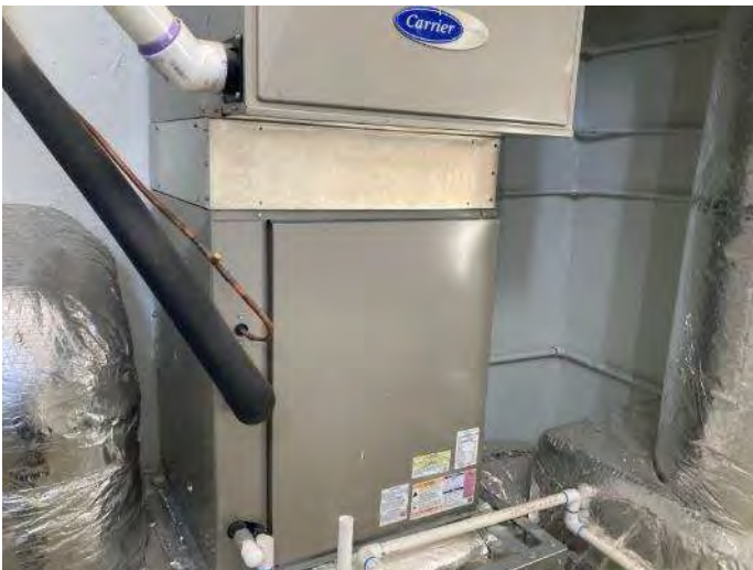
39. Split-AC system indoor fan coil unit
