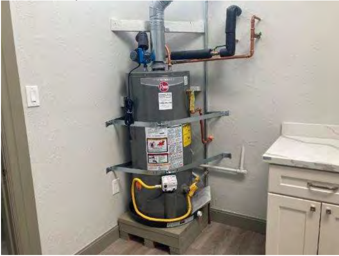
31. Gas storage-type water heater
