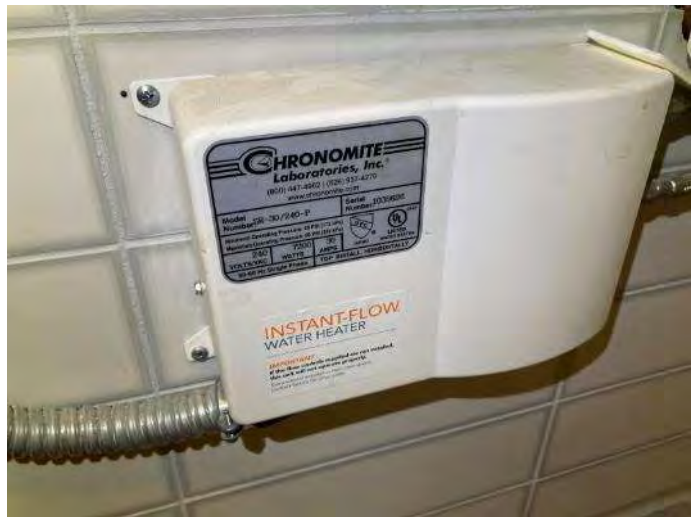
34. Electric instantaneous water heater in the first-floor bathroom
