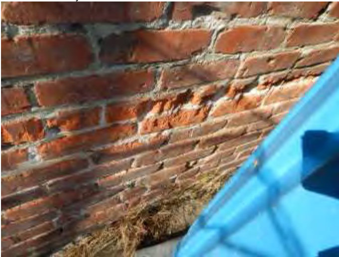
85. Deterioration of the masonry brick at the ground floor rear elevation
