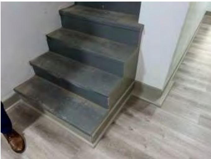
99. Missing guardrails on the basement stairs
