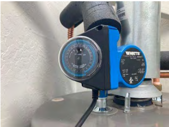
33. Timer controlled recirculation pump
