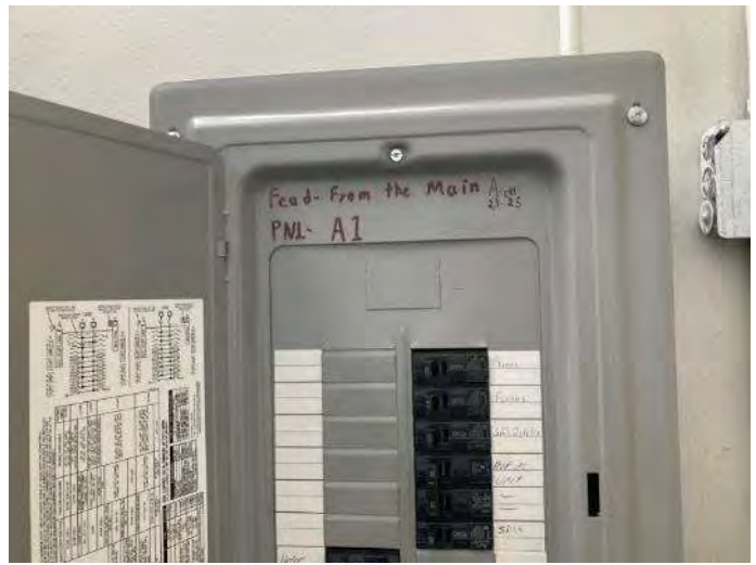
52. Electrical breaker in the furnace room at the roof level
