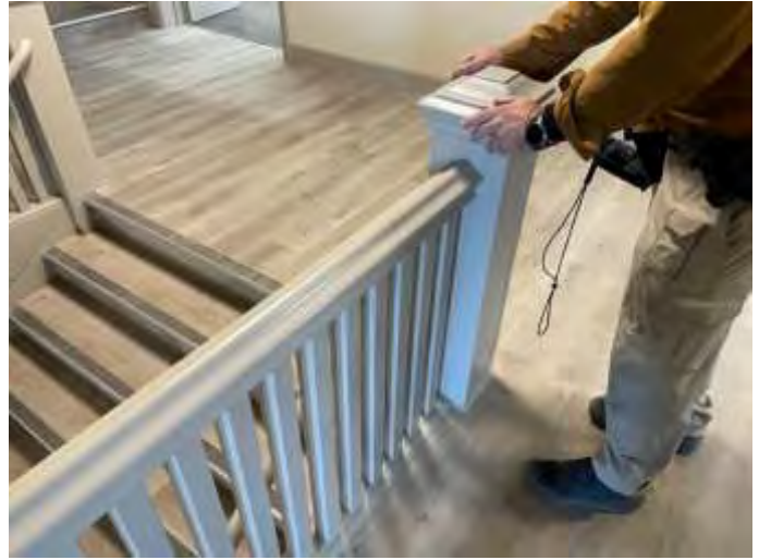
98. Guardrails throughout the subject property are too low and pose a fall hazard
