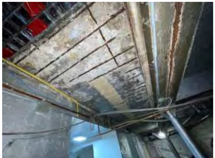
78. Exposed rebar was observed on the underside of the sidewalk in the basement
