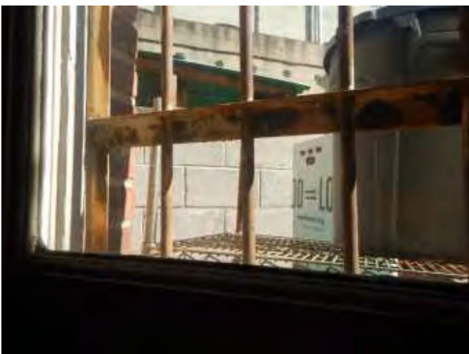
89. Rusted metal security bar at the ground floor rear elevation
