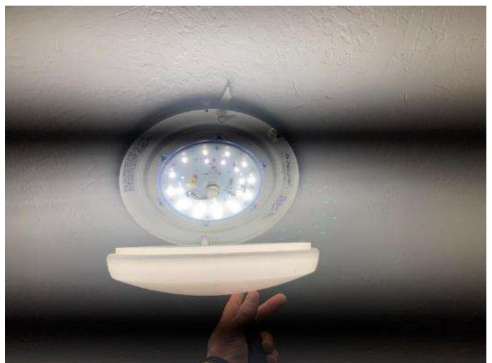
60. LED lighting in closet
