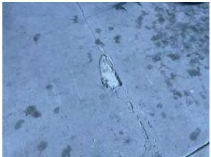
82. Deteriorating thin concrete poured sidewalk
