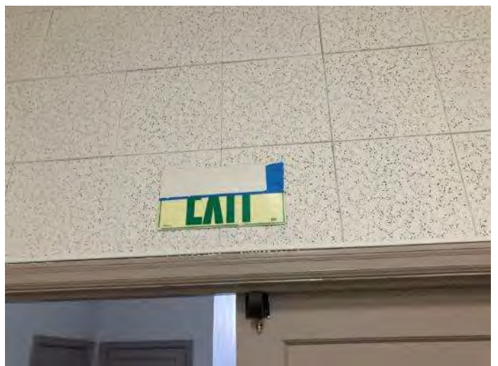
66. Broken exit sign in the 1st floor open area
