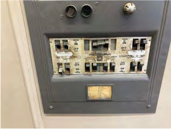
55. Old breaker panel in the 3rd floor open area
