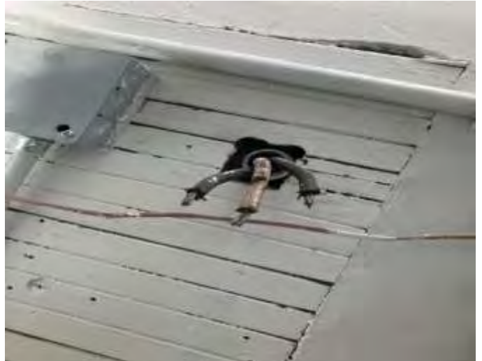
56. Exposed electrical wiring in furnace room on the roof level
