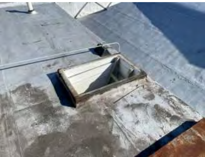
93. A proper roof hatch with safety rails needs to be installed
