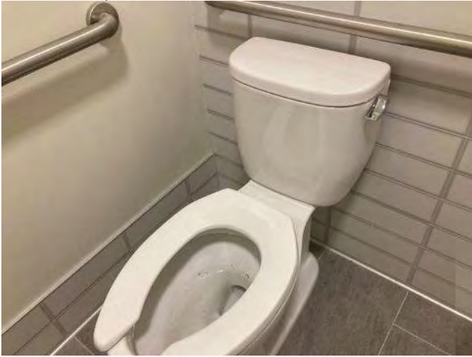
37. 1.28 gallon per flush toilet in first floor bathroom
