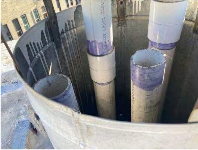
43. Gas furnace units' exhaust flue termination at the roof
