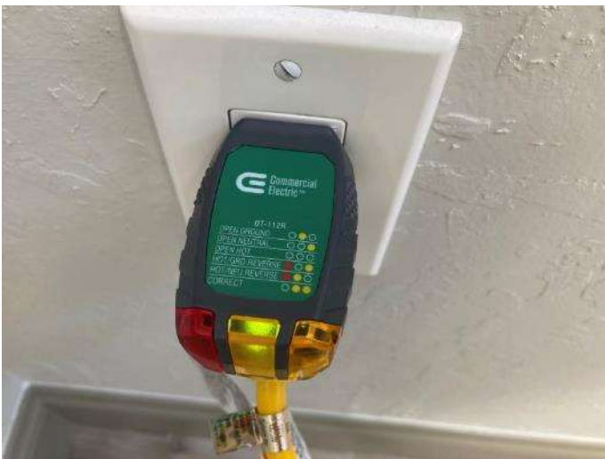
53. Functioning GFCI in the water heater room
