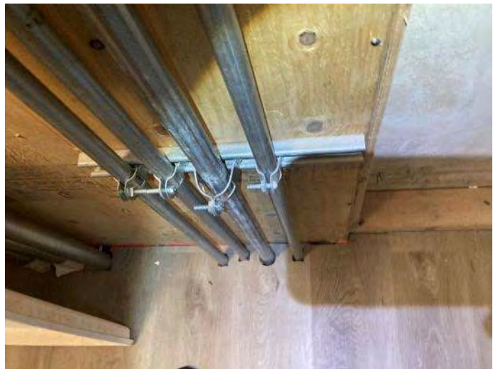
58. Uncaulked electrical pipes on 1st floor
