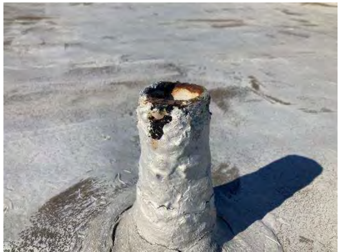
28. Cast iron sanitary vent
