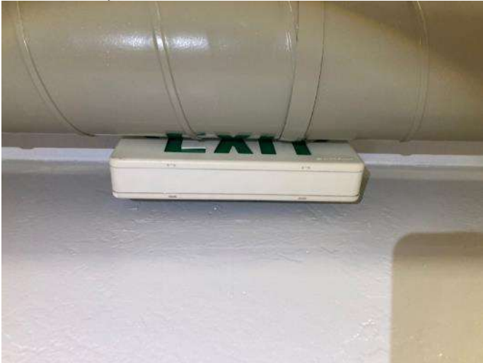
67. Exit sign in basement obstructed by HVAC duct
