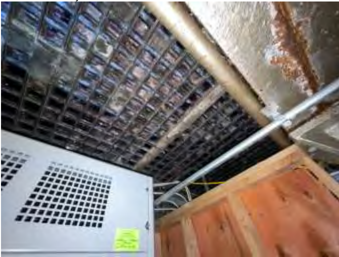
79. Exposed glass block was observed on the underside of the sidewalk in the basement
