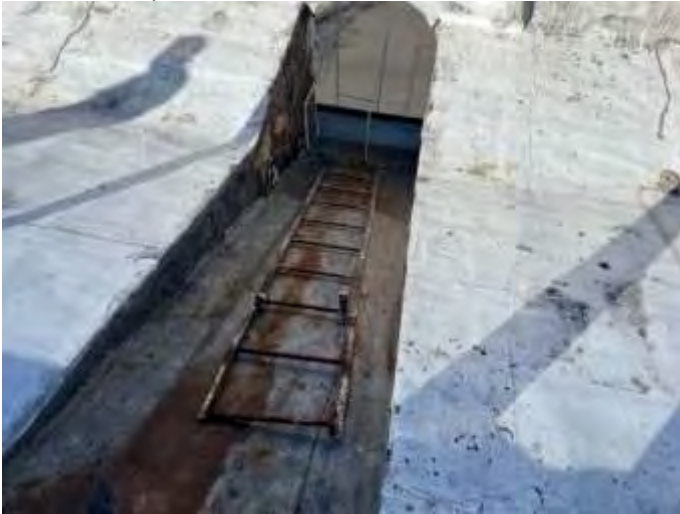
97. Unsafe fire escape access from roof
