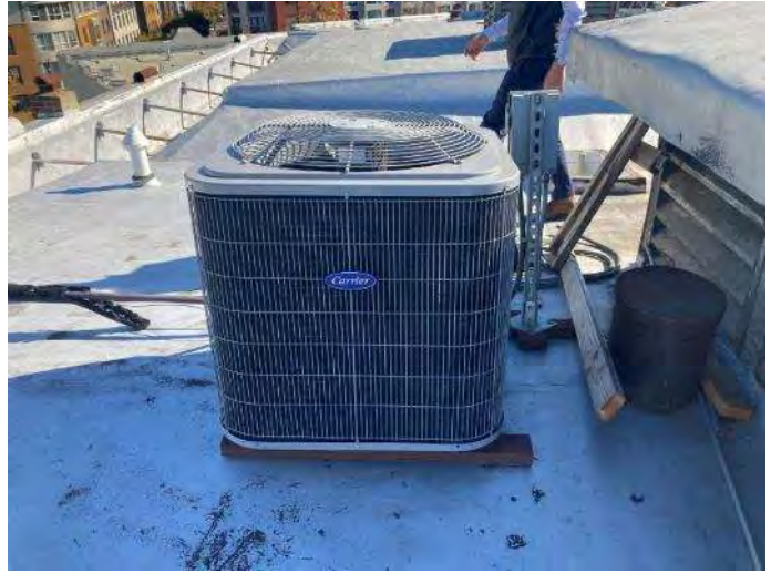
38. Rooftop condensing unit for split-AC system
