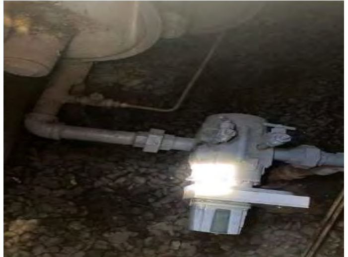
62. Gas meter in underground vault
