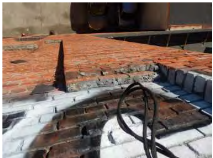
84. Deterioration of the masonry brick on the upper part of the rear elevation and graffiti
