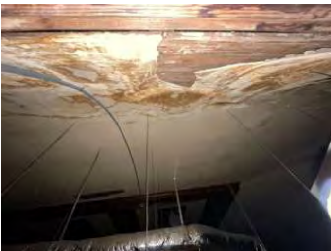
83. Moisture intrusion in the attic space above the auditorium
