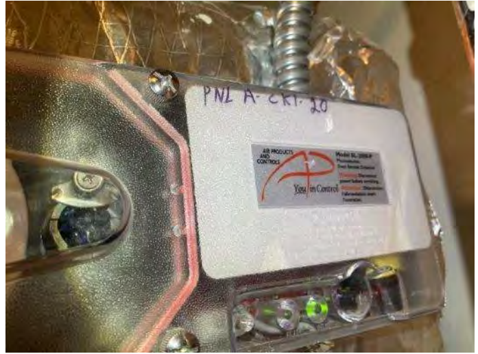
44. Gas furnace unit discharge duct smoke detector
