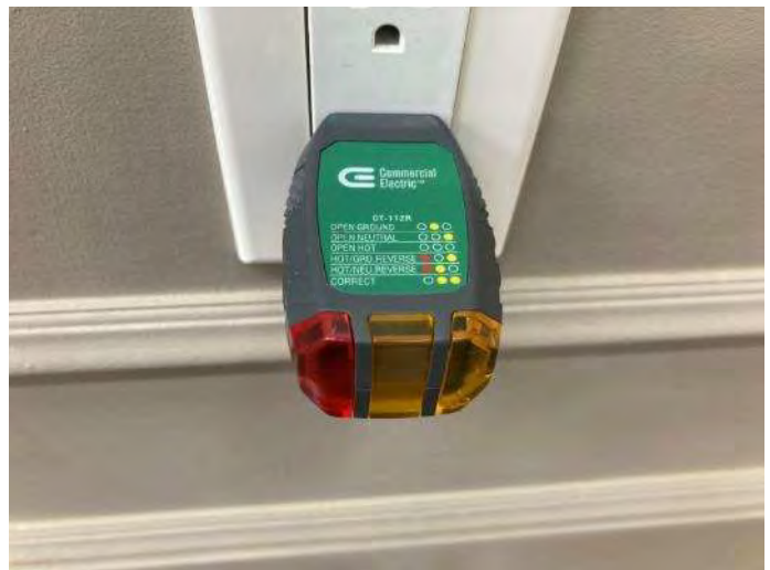
54. Open hot GFCI outlet in the 3rd floor open area
