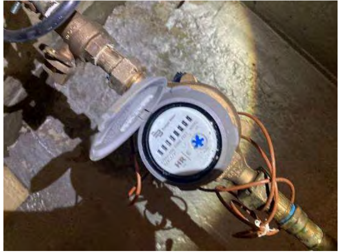
26. Water meter in the basement
