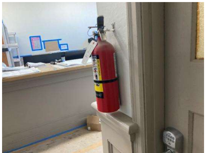
64. Fire extinguisher in the lobby office
