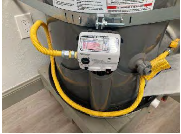
32. Floor pan for water heater
