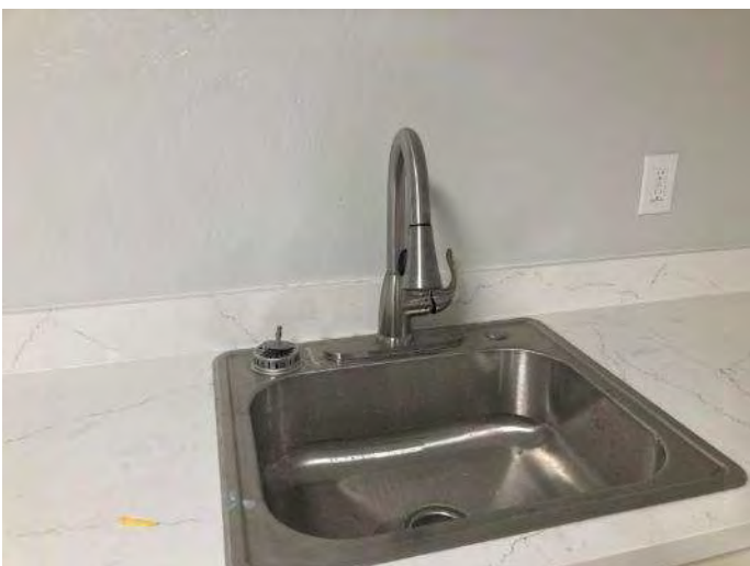
35. 1.8 gpm kitchen faucet in the basement
