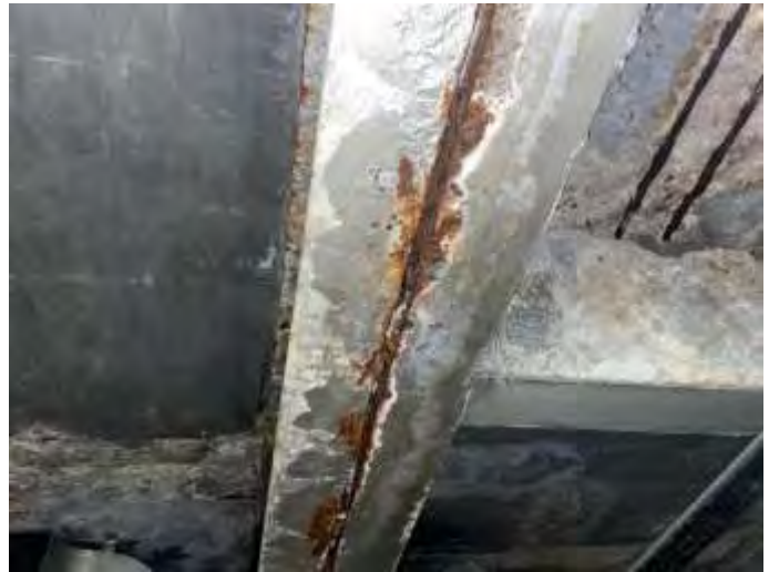
80. Rusted rebar and efflorescence were observed on the underside of the sidewalk in the basement
