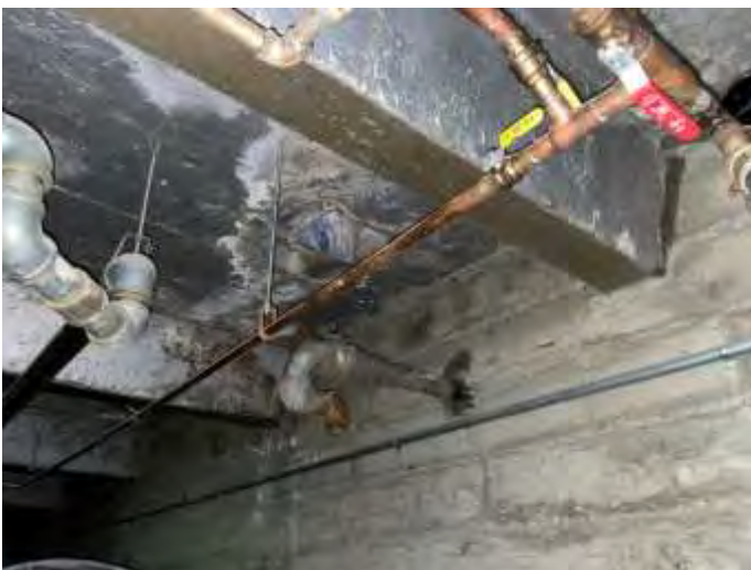
81. Moisture intrusion was observed on the underside of the sidewalk in the basement
