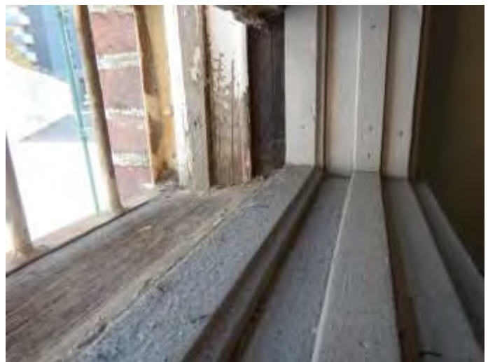
88. Rotted wood window frame
