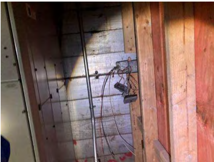
57. Exposed junction box
