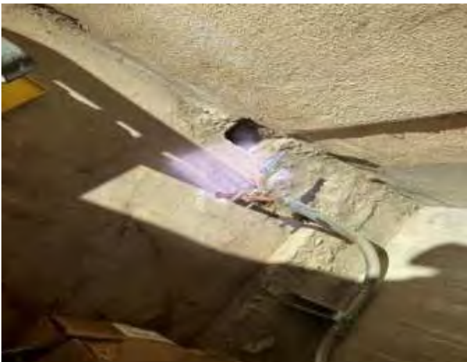
51. Copper wiring ground system
