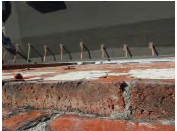
86. Close up of deteriorated mortar and brick coursing
