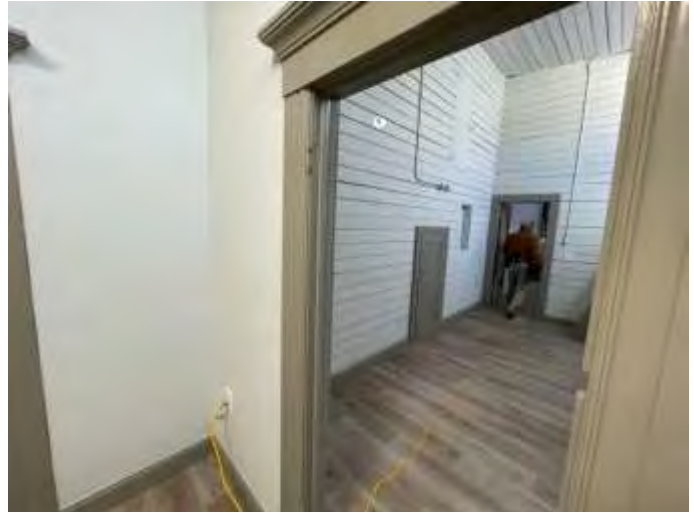
92. Missing door in the attic space
