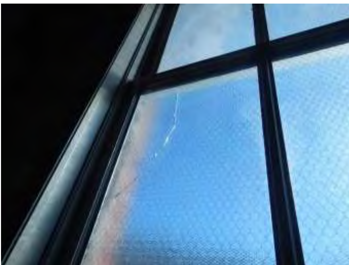
87. Cracked original window glazing
