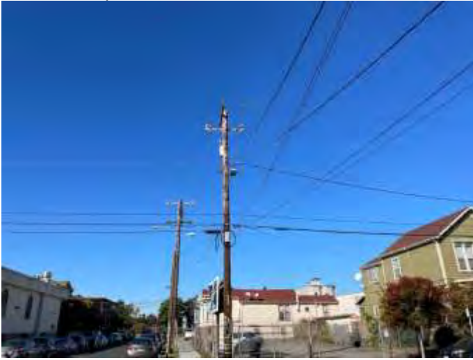
49. Pole mounted transformer
