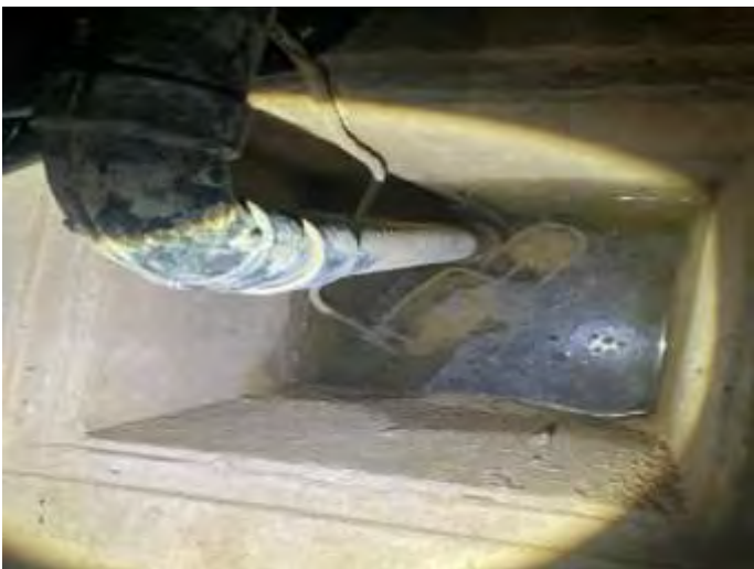
29. Sump pump in the basement
